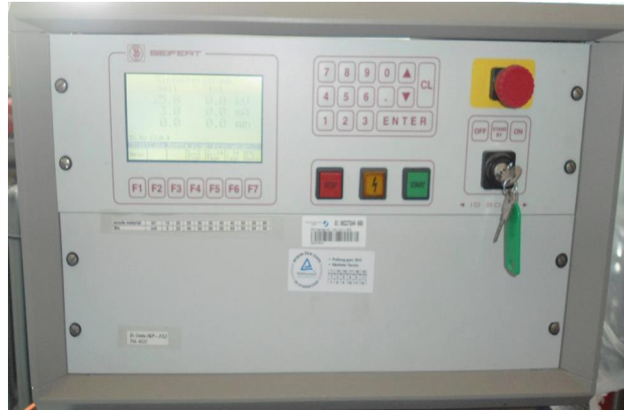
Figure 17: Operator panel of the high voltage generator [19].
